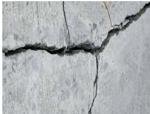
© stone crack, Fotolia #36569926
